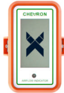
Figure 6 EXTRACTION NOT WORKING
